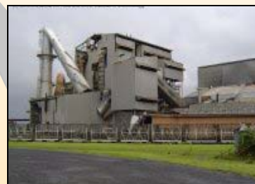
Sugar mill damage
